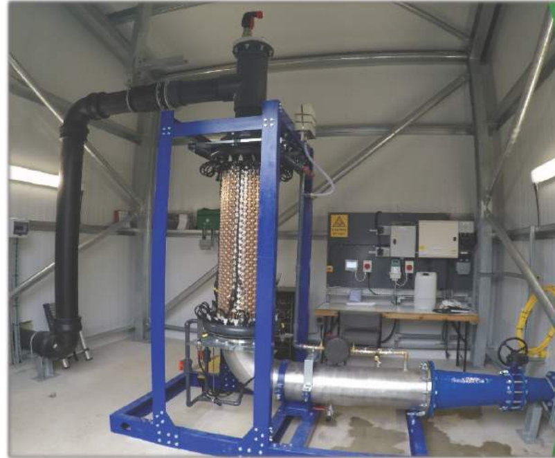
BIO-310 UV Reactor installed at Cumwhinton WTW
